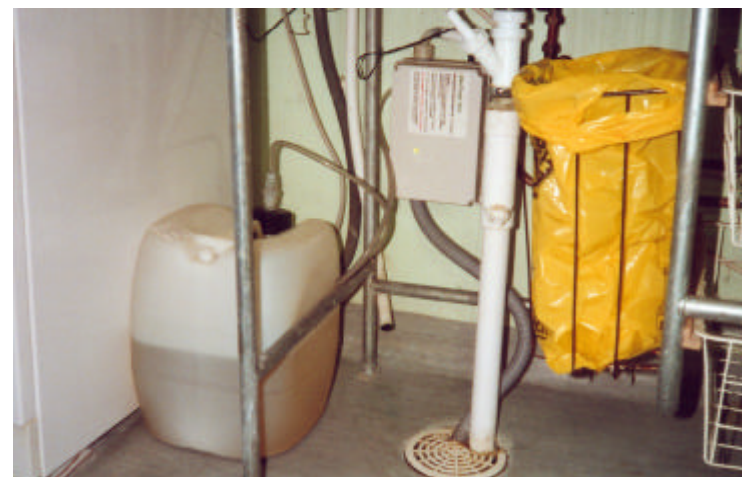
Figure 19. Equipment for chemical precipitation installed within the house.
